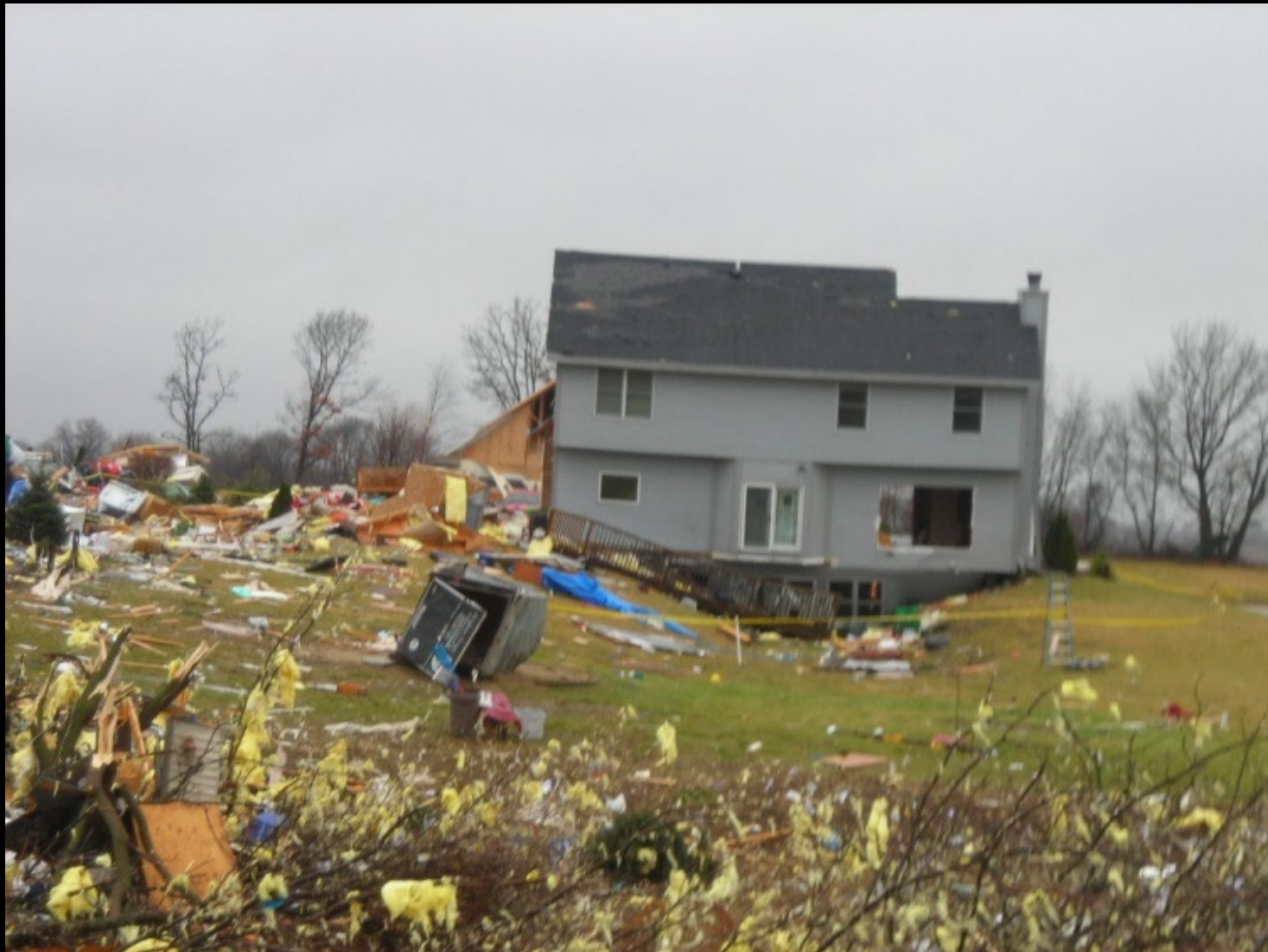
A neighbor to the west. Their house was three feet off the foundation.
