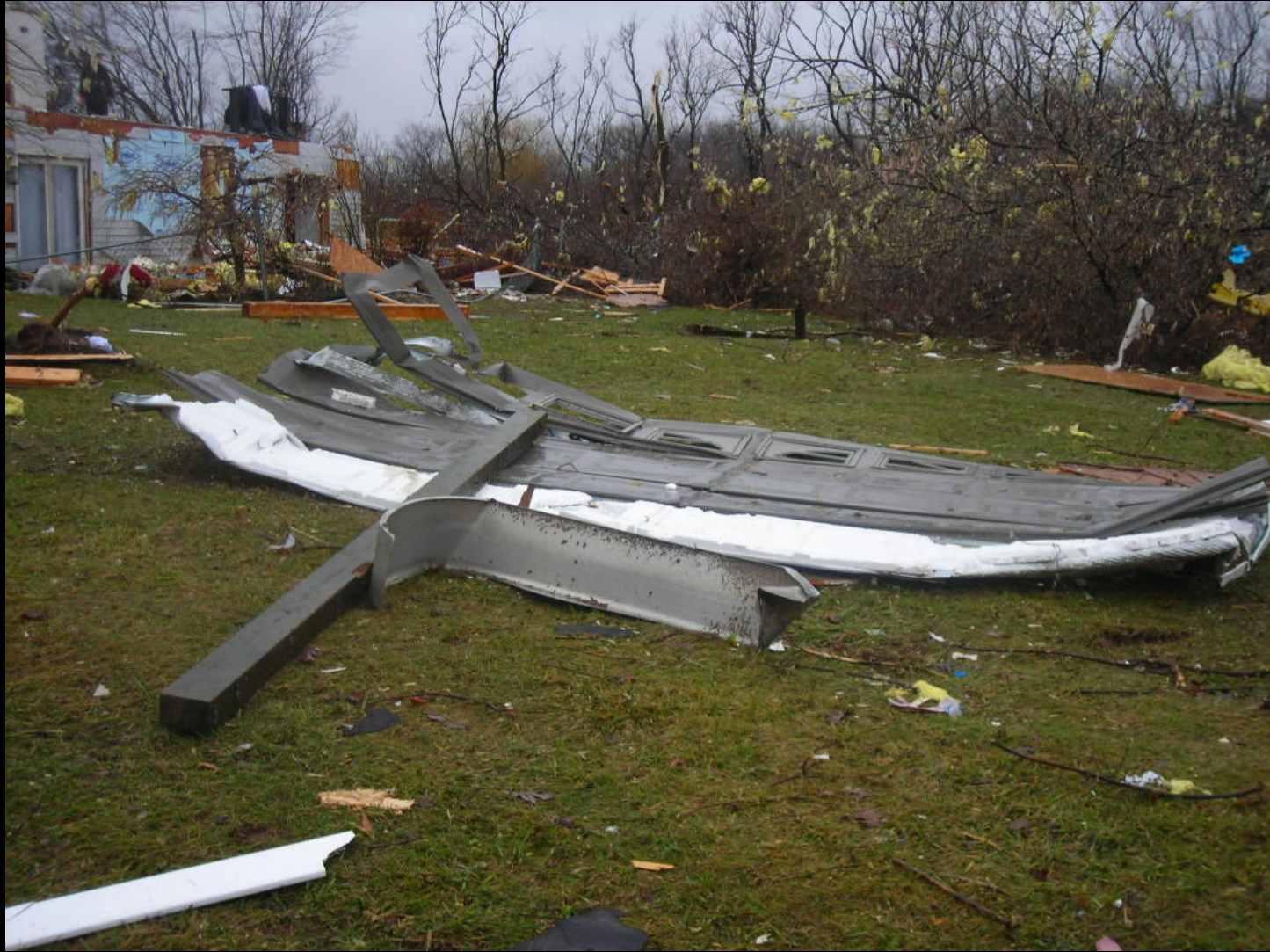
The neighbor's garage door laying in the yard. Note the lowest level of the house is still intact.
