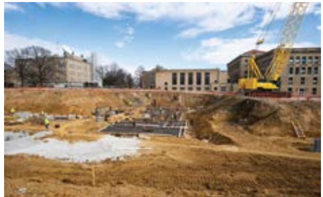
A 24-hour streaming site is available to watch construction on the Center for Performing Arts building at bit.ly/WIUCPASTREAM .
