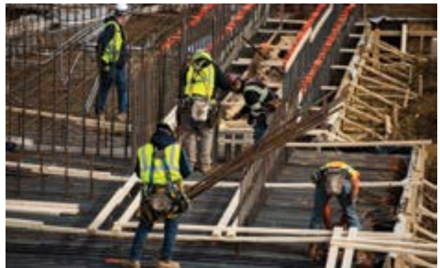
The Center's Great Hall Auditorium is beginning to take shape below ground level.
