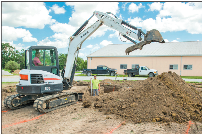
Construction crews broke ground in July for the Western Illinois University School of Agriculture's greenhouse project. According to School of Agriculture Director Andy Baker, in the initial phase, two 16 ft. x 48 ft. greenhouses (with a connecting hallway) are being built near the University's Livestock Center.
